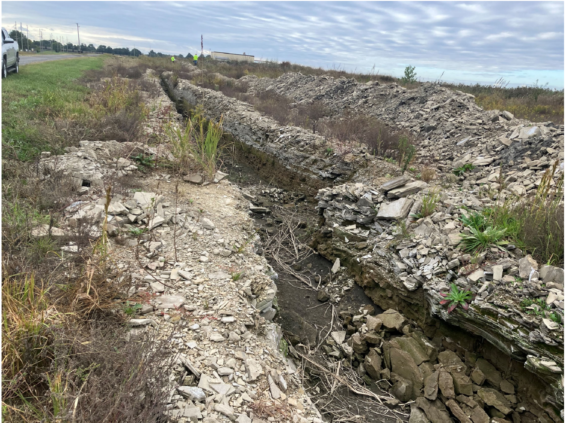
Photo of Excavation of Drainage Ditch Along East Berm of Fly Ash Pond. Note solidified fly ash in upper 5 feet. (10/13/2023)
