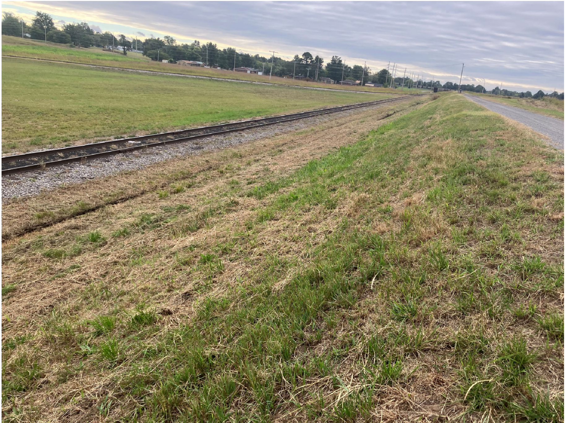
Photo of Sloughing Along Drainage Ditch, East Berm of Fly Ash Pond. Note that berm slope and road appear unchanged. (10/13/2023)
